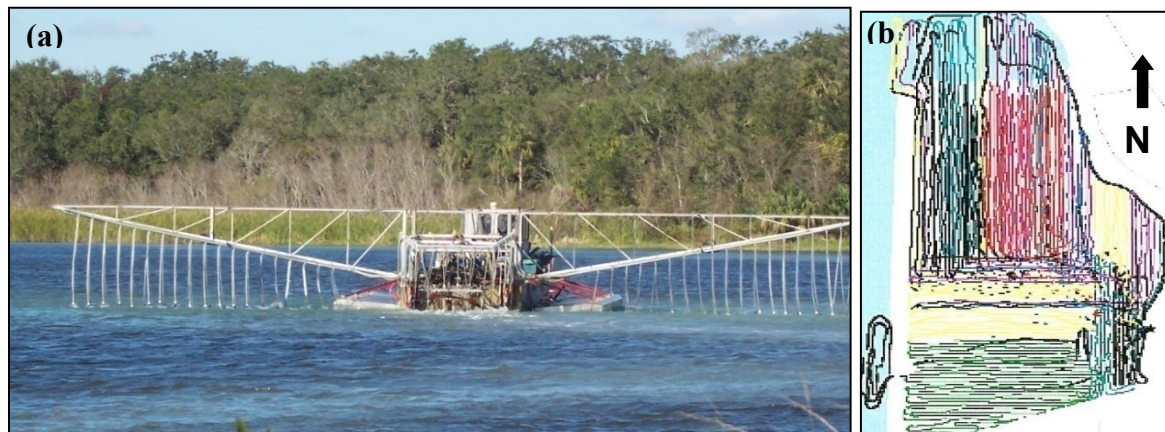
Figure 20. (a) Alum delivery system from Sweetwater Technology. Liquid alum was injected in a swath from hoses attached to each boom arm. (b) Routes of the alum barge system (recorded by GPS). Each color represents a different day of application.
