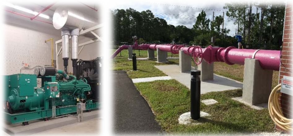
A utility generator at a reverse osmosis plant, Palm Coast Utilities, left. Reclaimed water facility in Daytona Beach, right.
