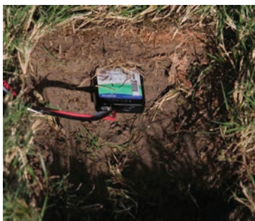
Soil Moisture Sensor Installed
